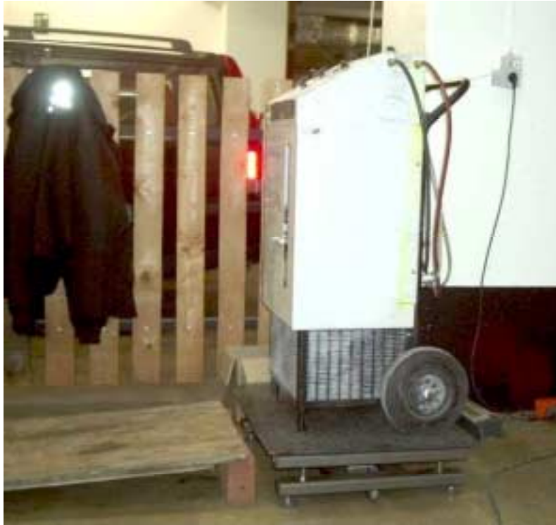
Figure 14: A recovery station Waeco RHS 650 on the scale before and after the recovery operation.
